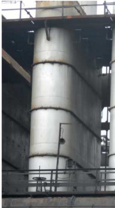
PRIMARY GAS COOLER
