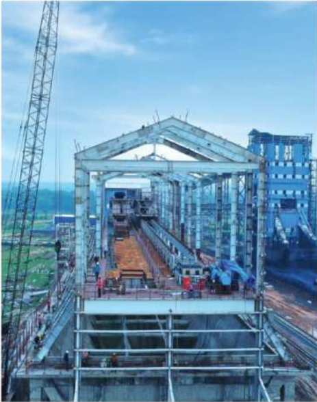
COAL HANDLING PLANT AT PAKRI
