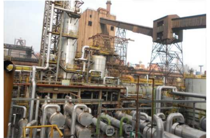
BENZOL ABSORPTION & DISTILLATION PLANT AT SAIL - DURGAPUR
