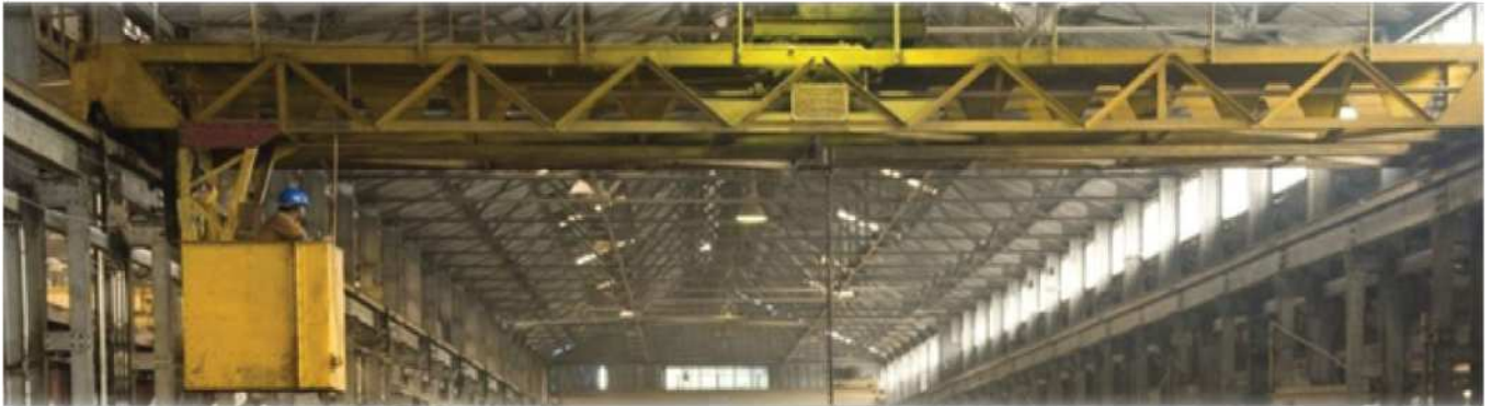
EOT CRANE (HANDLING MATERIALS)
