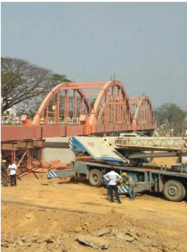
FABRICATION & SUPPLY OF STEEL ARCH BRIDGE FOR NCC AGARTALA, KATAKHAL FLYOVER PROJECT
