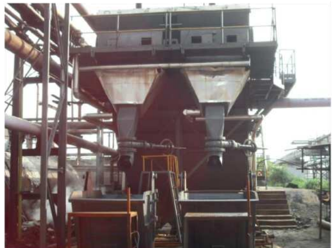
TAR DECANTER FOR COKE OVEN BATTERY, SAIL - DURGAPUR
