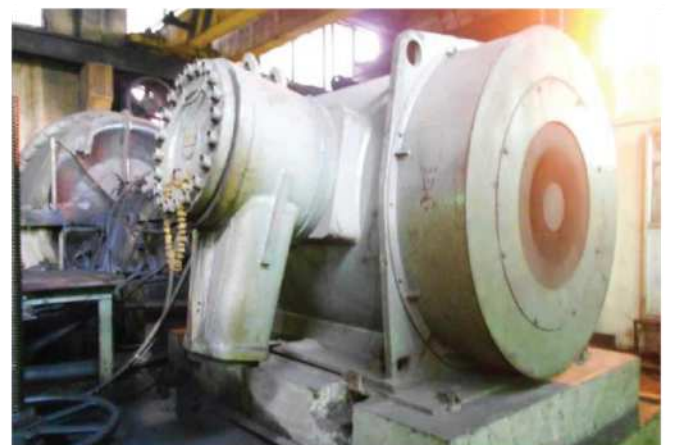
ELECTRIC EXHAUSTER FOR COKE OVEN BY- PRODUCT, SAIL - DURGAPUR
