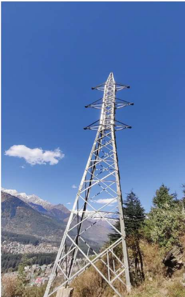
66 KV D/C TRANSMISSION LINE AT MANALI (LINE LENGTH - 9 KM) CLIENT- HPPTCL
