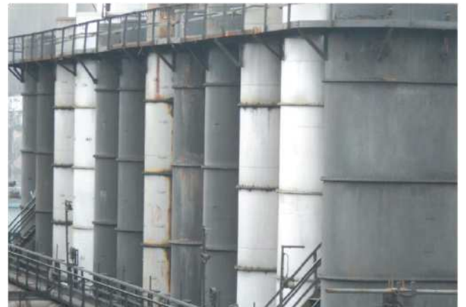
SAIL, DSP PRIMARY GAS COOLER
