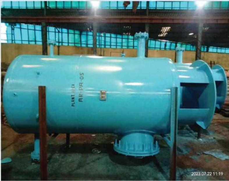
AIR RECEIVER (PLANT AREA)
