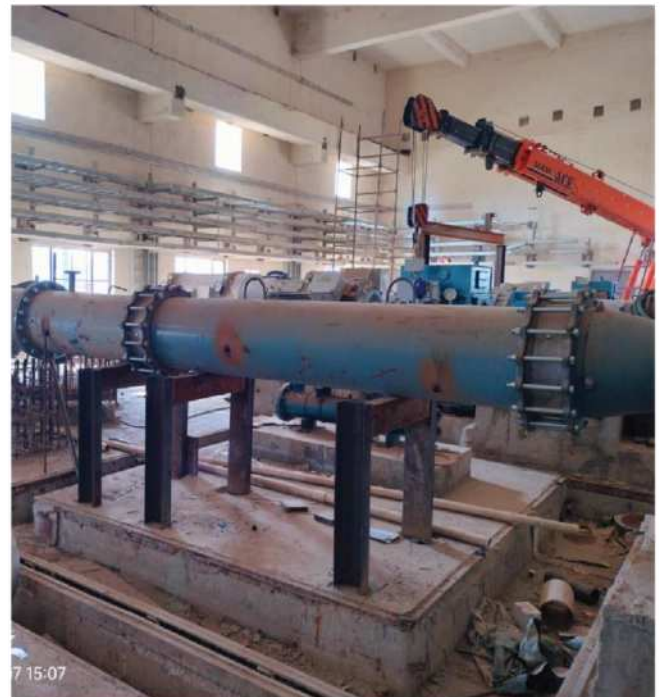
ASH SLURRY PUMP HOUSE AT YADADRI
