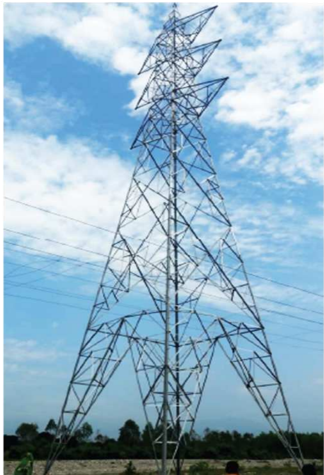
132 KV D/C TRANSMISSION LINE FROM RANIKHET TO BAGESWAR - (LINE LENGTH - 43 KM) CLIENT - PTCUL, UTTARA- KHAND
