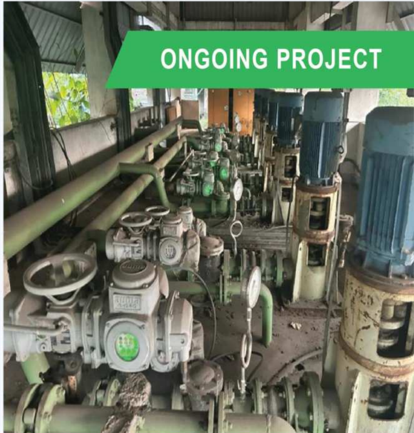
DVC - BOKARO (PRE TREATMENT AND ETP PLANT)
