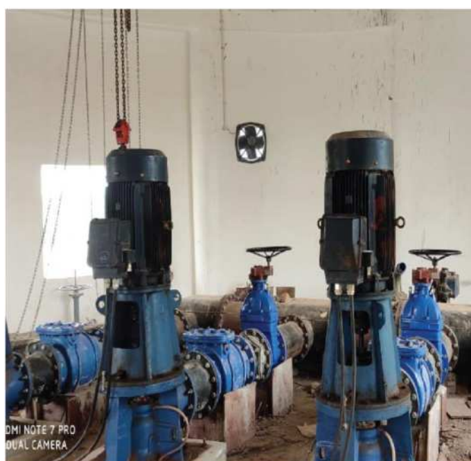
INTAKE PUMP HOUSE WITH VERTICAL PUMP
