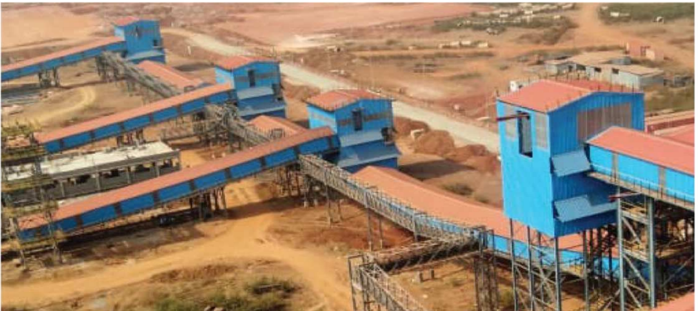
NMDC, NAGARNAR PROJECT: RMHS SINTER ROUTE & COAL ROUTE
